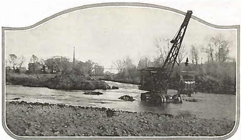
Building of more miles of good roads per dollar is only one of the functions of the State Highway Department. Here is shown a dragline machine used in excavating new river channel near Del Norte.
