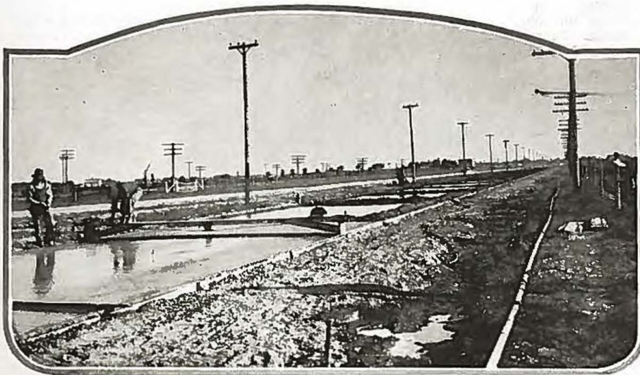
Showing method of "curing" concrete employed on paving project near Brighton. Water is pumped into dikes around each slab.
