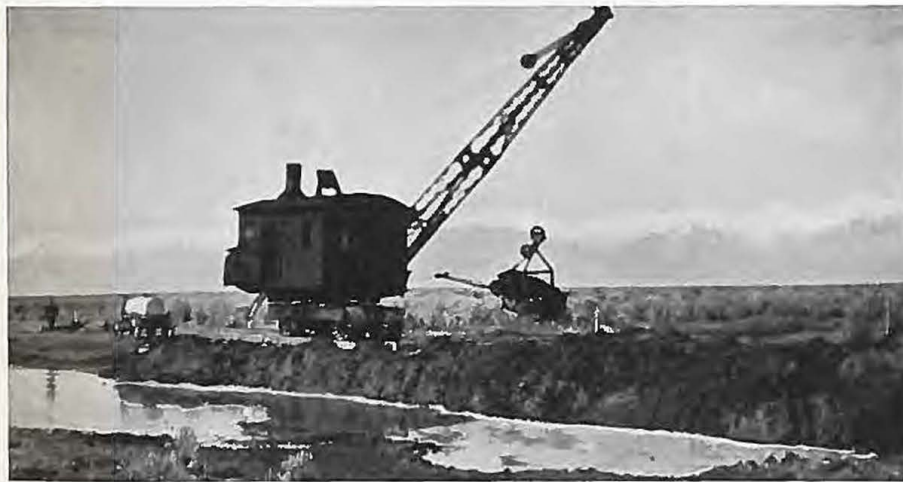
Picking a road up out of the mud with a droyline between Hooper and Mineral Springs.
