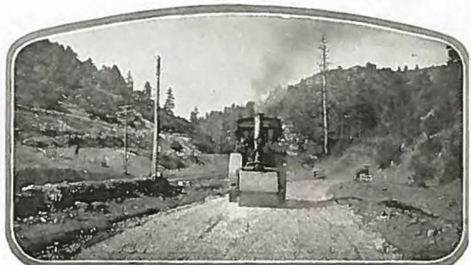
A giant steam roller in action on the lower course of gravel project being constructed with Federal Aid funds on the Durango-Manco Highway.
