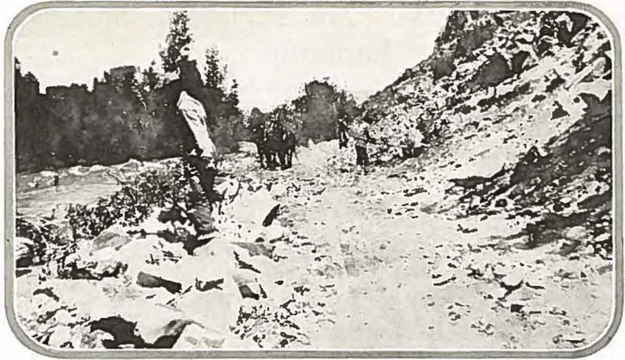
On the way to Cumbres Pass. View shows part of road crew at work widening rock cut near Boyle's Bridge on State Highway No. 67, along the Conejos River.
