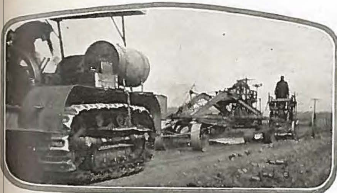
Modern machinery used in making better roads in the San Luis Valley. Picture taken below town of Adler in Saguache County.
