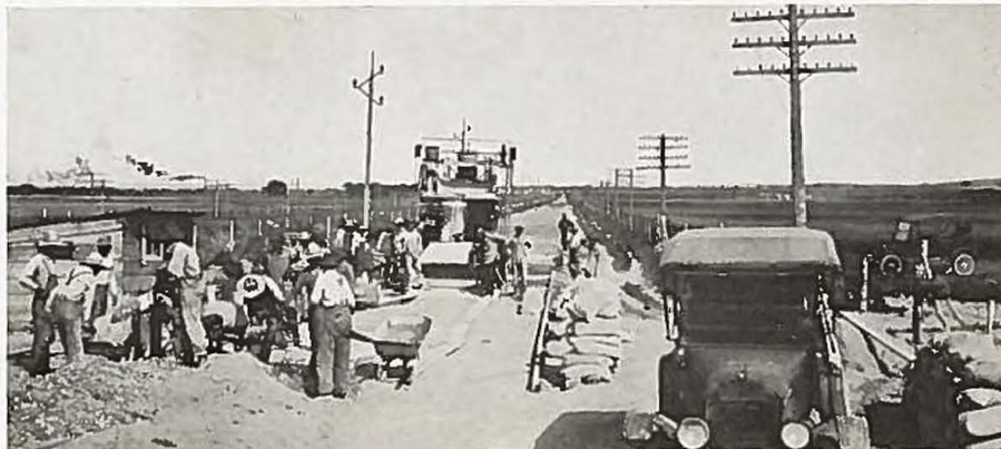
Concrete mixing crew at work on Santa Fe Trail west of La Junta in Otero county.
