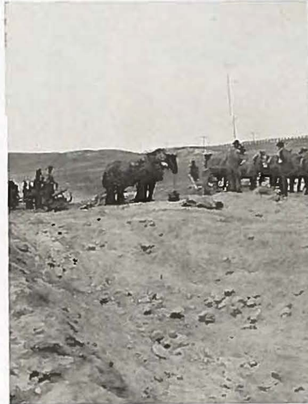
Showing grading work on Highway No. 30 in Lincoln county between Colorado Springs and Limon.
